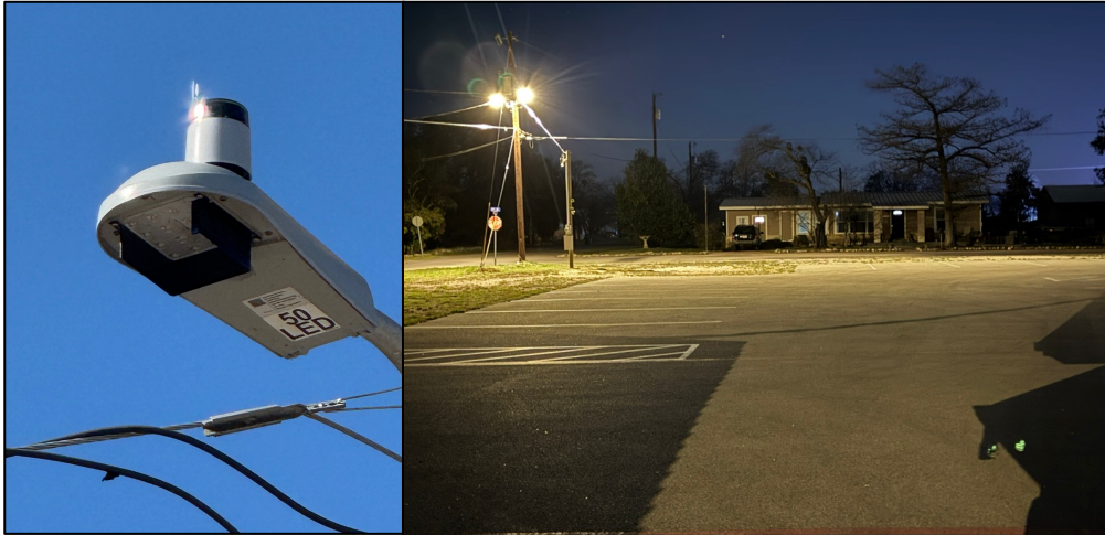
Streetlight with Glare Shields Installed
